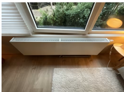
Radiator i stue.
